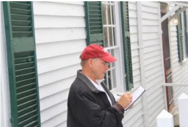
Bill Remsen, a registered architect, is assessing the firehouse windows. Bill lives on River Road and recently joined the History museum steering committee.
